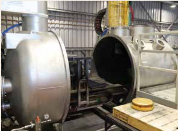
One of the new PAM units at the refinery.
